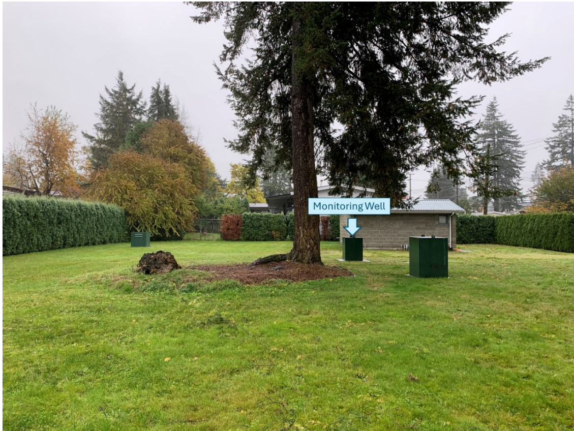
IMAGE | CWD DESIGNATED MONITORING WELL - MW 6-59.
