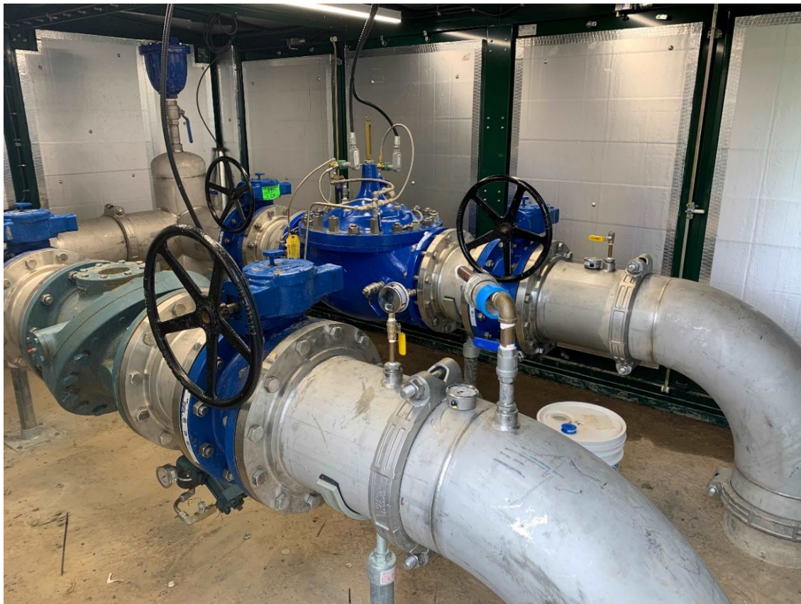
IMAGE | WATER INFRASTRUCTURE AT THE RESERVOIR SITE.
